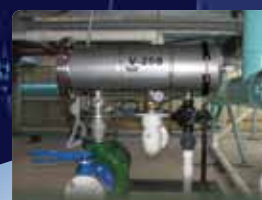
COOLING TOWER Medical-Melbourne
