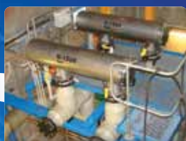
SEAWATER FILTRATION Offshore Atlantic
