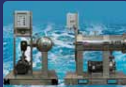
SEAWATER FILTRATION Offshore Platform North Sea & South China Sea
